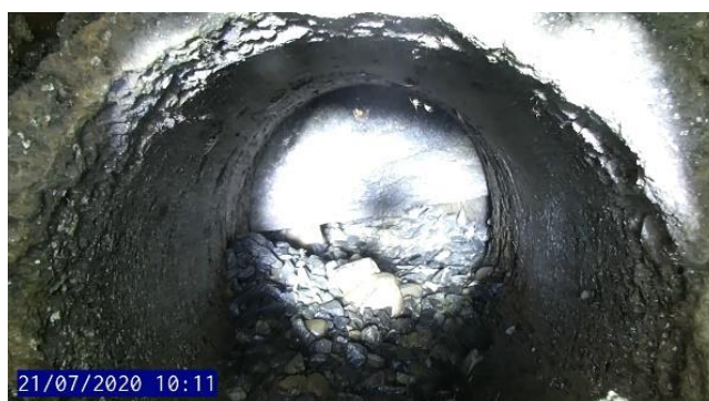
Examples of blocked pipes
